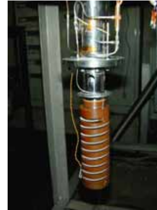
Still & Heat Exchanger
